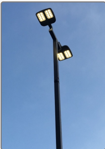
Street scapes lighting
